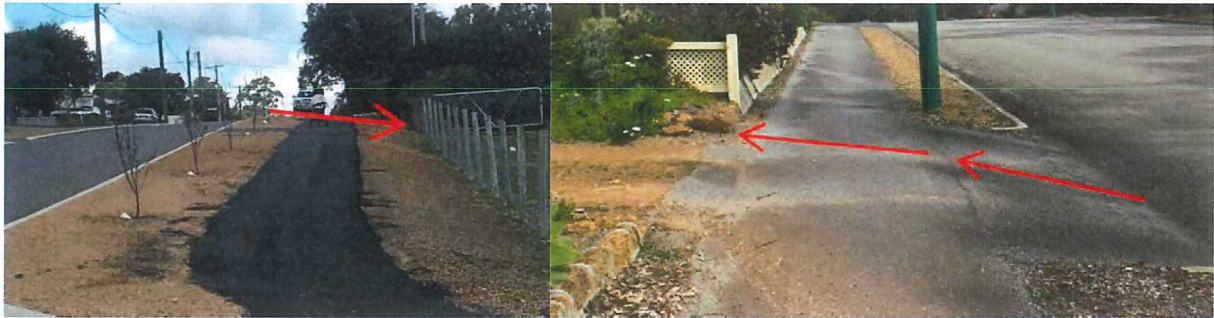
Photos 19 and 20: Significant down and up crossfall grades on verges
