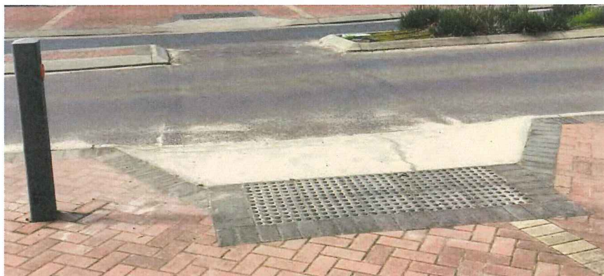
Photo 24: Concrete and paved Pram Ramp with Tactile Ground Surface Indicators (TGS) and consistent with current standards (Lowood Road)
