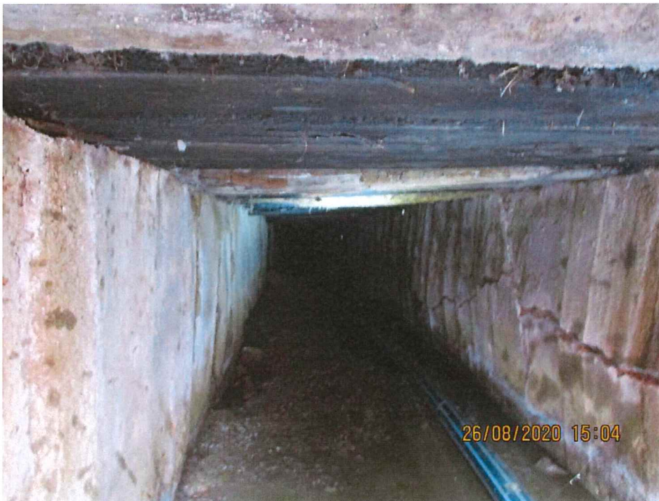
Looking eastwards under track through culvert system. Note rotted and cracked timber, cracked and bowing side walls. Some grass roots can be seen growing down through the lid.
