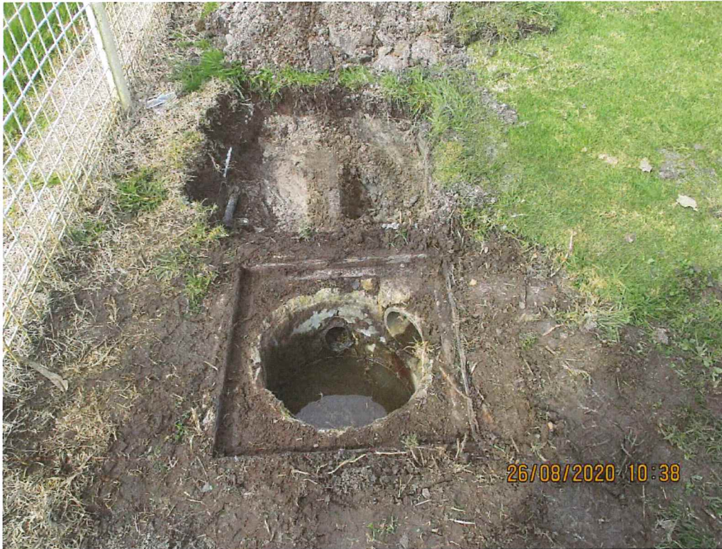
Pavillion roof water collection sump looking south. Note inlet of downpipes is higher than inlet of subsoil. Outlet from sump (not shown) is higher than subsoil piping.
