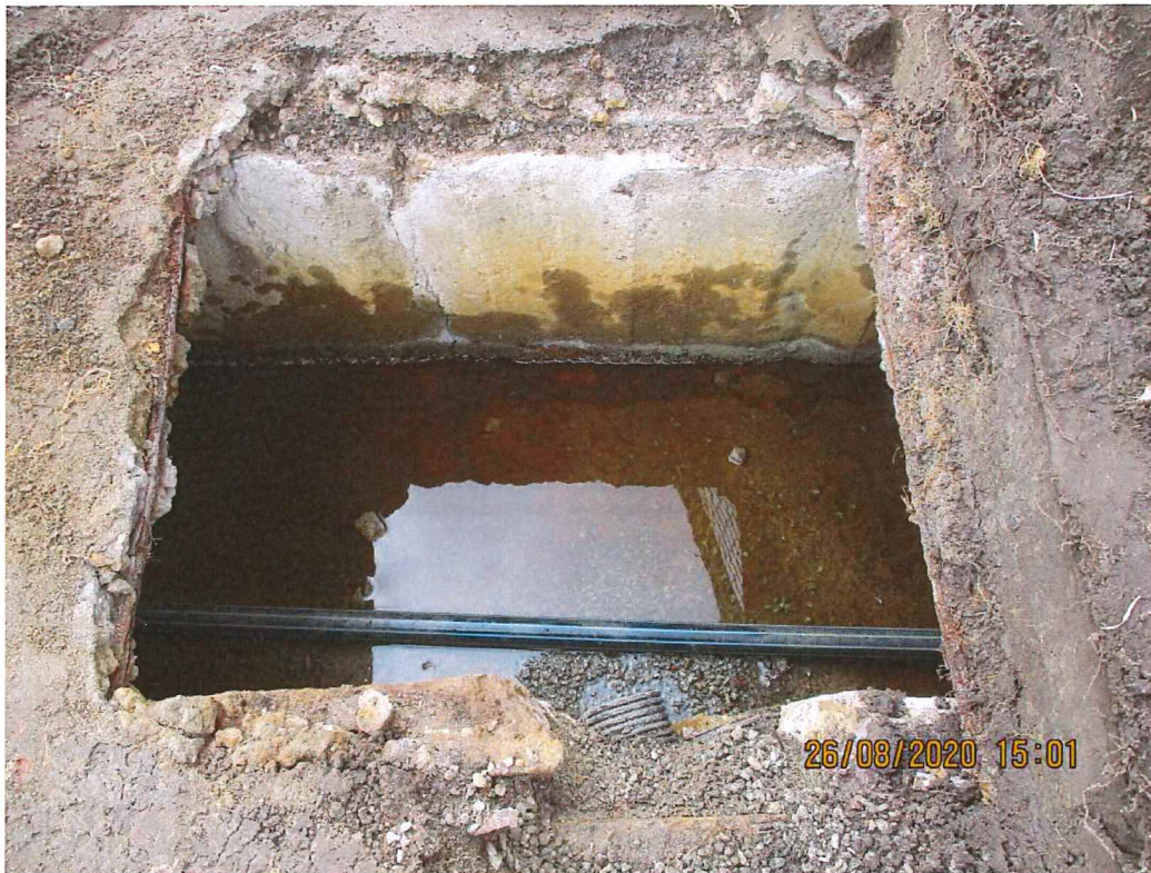
Western side of track where under track culvert begins. The subsoil system from the pavillion area is supposed to terminate here but note that there is no water flow.
