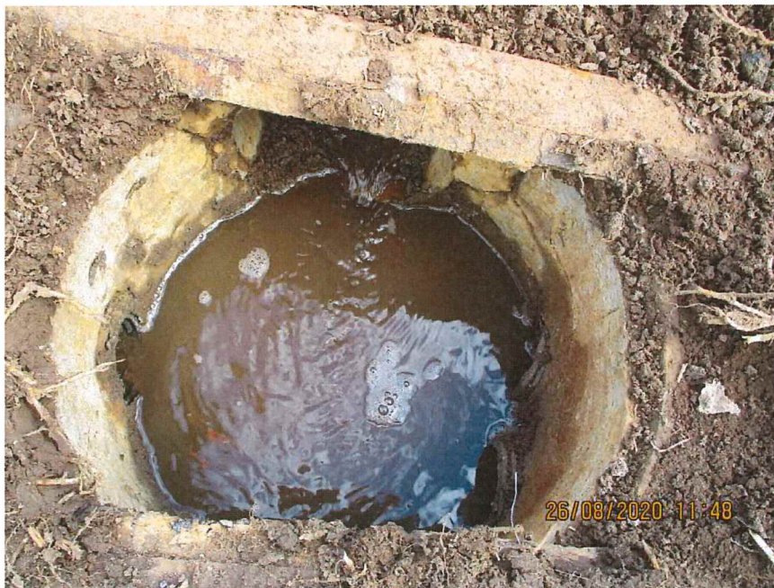
Ag Shed water collection sump. Note that LHS subsoil pipe leads back towards Pavillion and is lowest point in the sump. ie Flow is backwards to what it should be.
